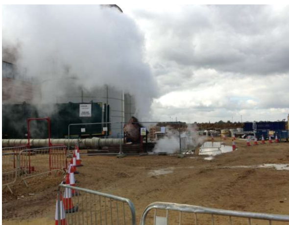
A Steam Blow test in progress
